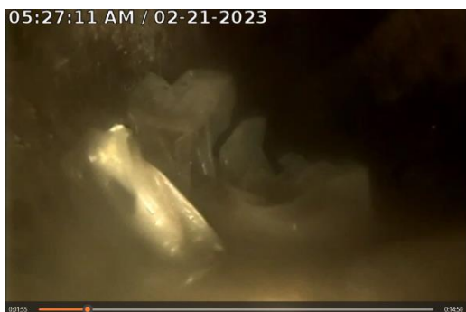
Toilet paper evident at 38'.
